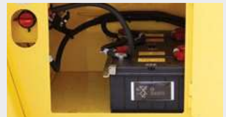
Battery compartment with lockable battery disconnect switch
